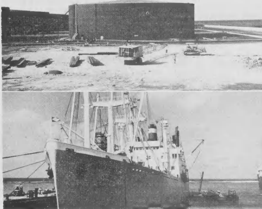
PREPARATIONS FOR the construction of Lago's new No. 3 Finger Pier are rapidly appearing on the refinery scene. Near the fire training grounds a sand blast area is being readied for the contractor, Raymond Concrete Pile Company. The Santa Sofia brought in some of the pilings needed, and at the barge dock waits one of the contractor's huge cranes.
